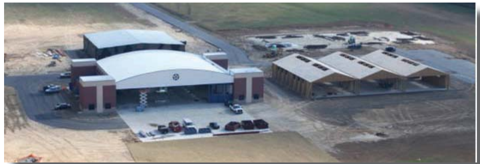
Aerial view of the museum while the WWI hangar is under construction
